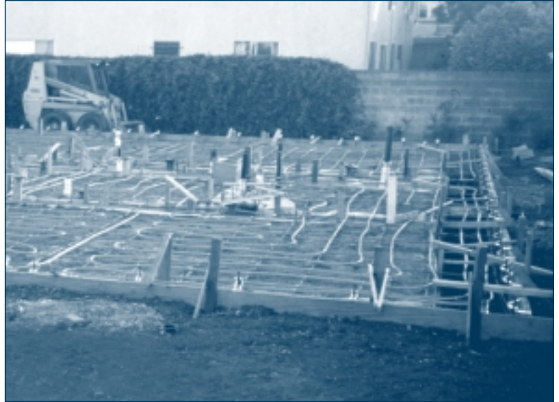
Radiant Floor Heating
